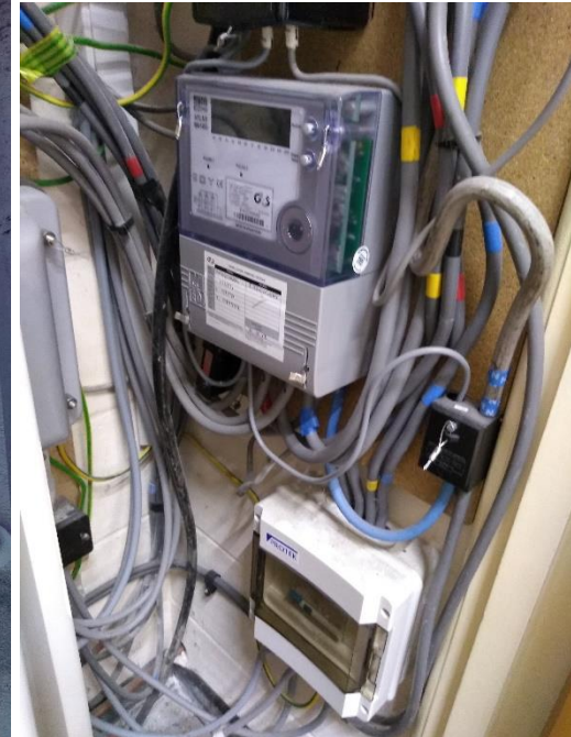
Primary Switch Board 1
