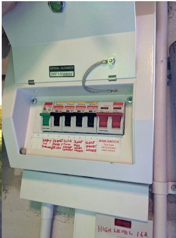
Secondary Switch Board 1
