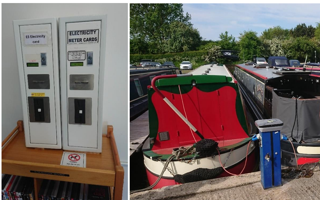
183 Electricity meter cards dispenser and electricity (and water) unit at Cowroast Marina.
